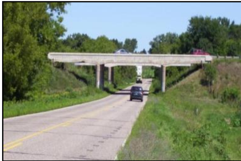
Aging bridges with substandard clearance over 100 th Street
